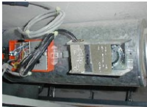
Existing volumetric flow controller box:
